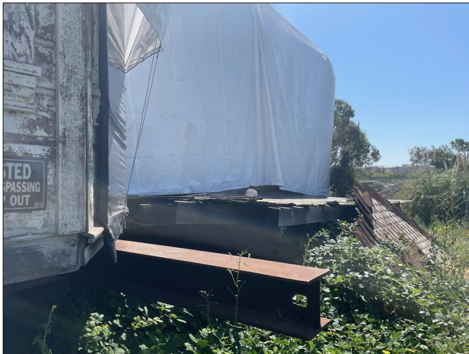
Interior or porch floor exposed and partial roof with shingles on the ground.
