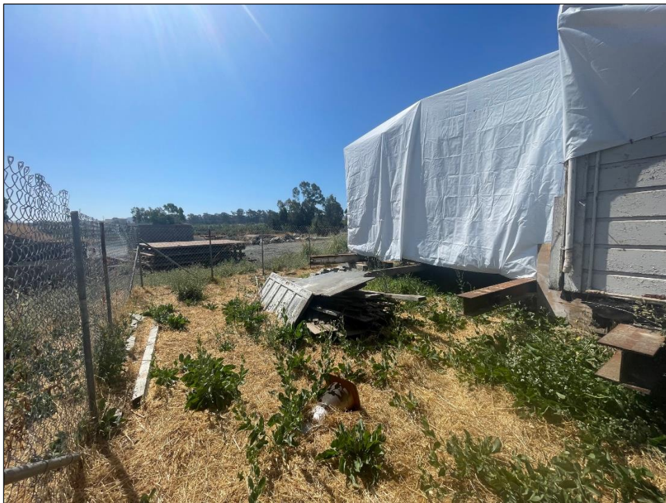
Side of subject structure with removed doors on the ground.
