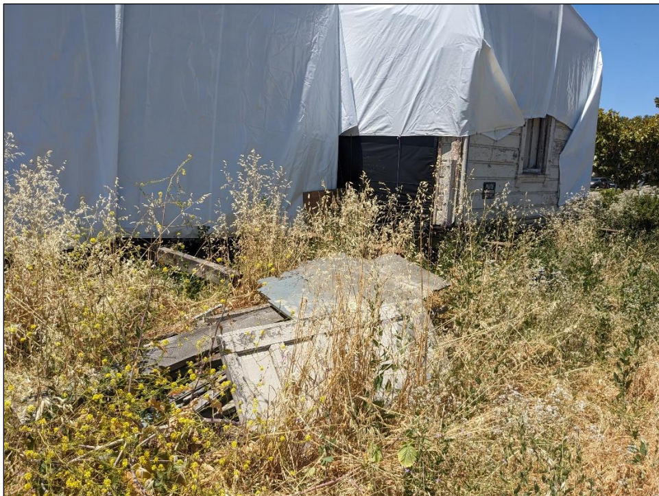
Door and siding detached and outside of the subject structure. Prior to August 2024.
