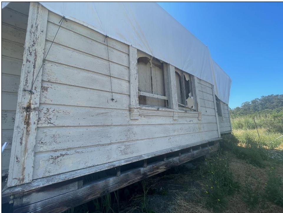
Side of subject structure with three windows partially exposed and flooring exposed.
