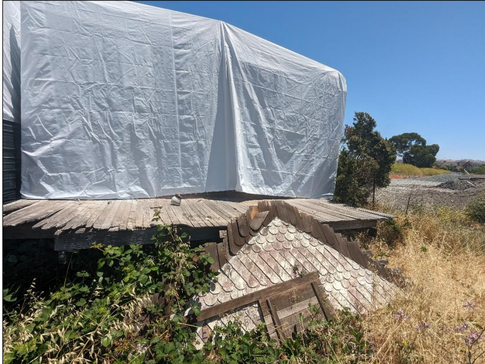
Partial roof with wood shingles detached. Prior to August 2024.
